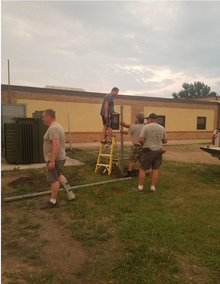
Above: The fence was also put up around the electrical boxes. Lion Jon Ellerbusch is shown on the ladder setting a corner pole as Lions Randy Bachmann and Matt Bailey assist, and Jack Foster walks to help on the other side of this project.
